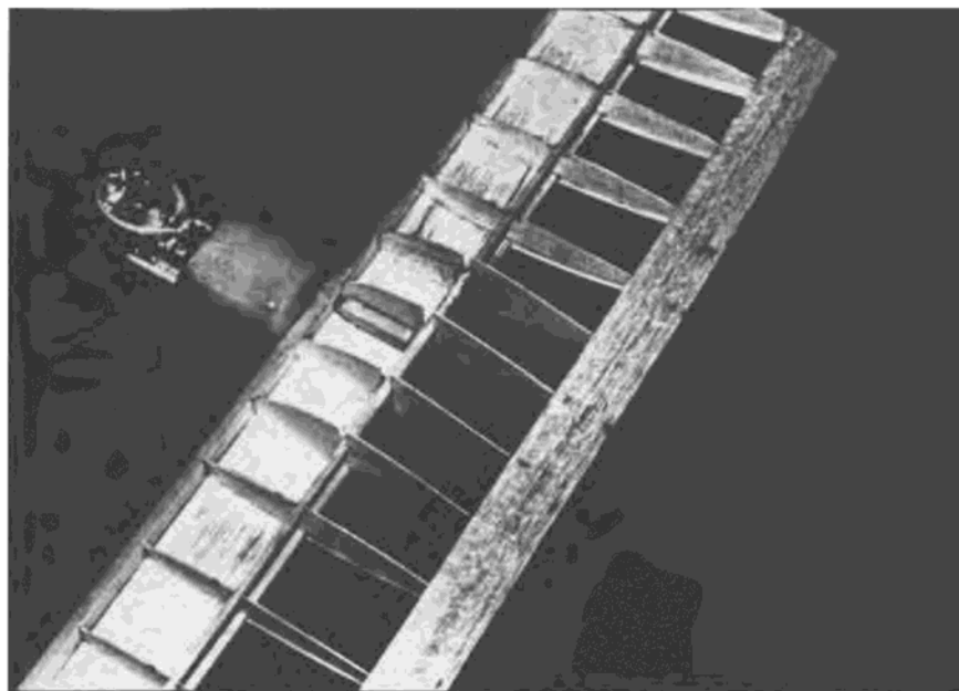
The engine mounts and plywood shear webs installed. Note the fuel tank temporarily installed to ensure adequate clearance. Be careful installing the rear halves of the center ribs to get the bottoms flush with the lower spar. This will allow the lower sheeting to fit properly.
