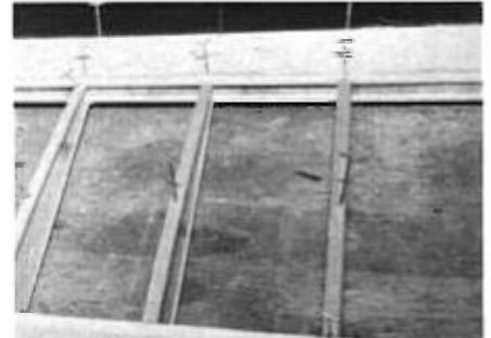
Cap strips and rear top sheeting are shown in this view. Pin down surfaces to be glued until they are set to insure a good glue joint.
