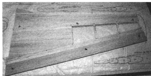
Although fully symmetrical, the wing is built on a flat surface. Here, the bottom sheeting has been pinned to the plans over wax paper.
