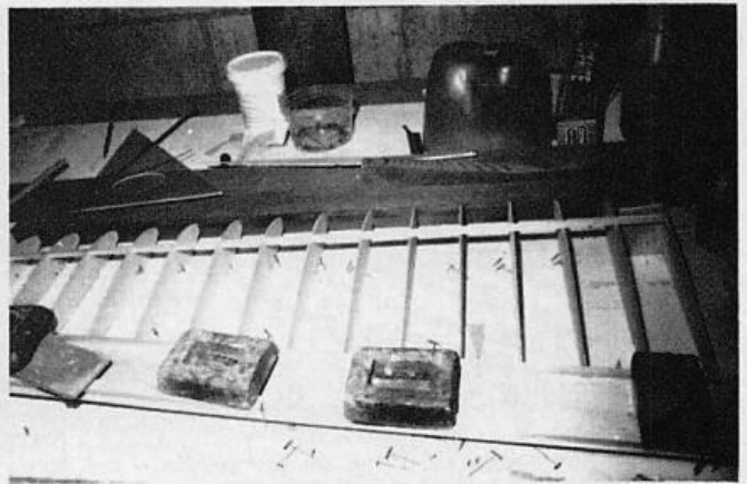
Wing is framed up with washout piece under T.E. Only top T.E. sheet applied here.
